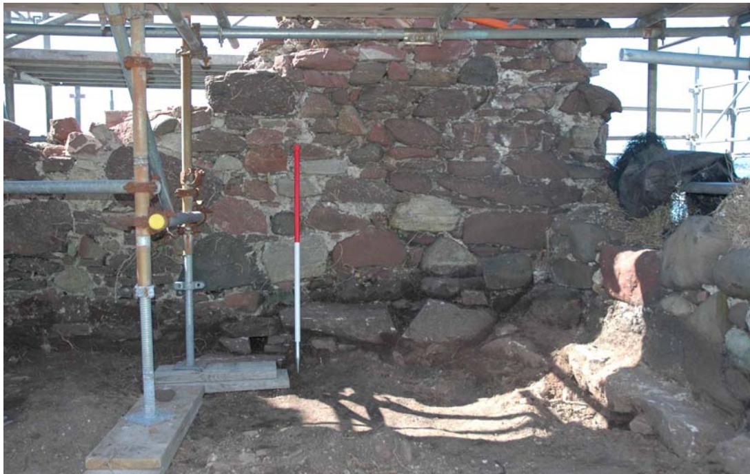
Plate 65: Interior of north corner of Lower Roof showing the drain (630) to the left of the pole and the scarcement to the right.
