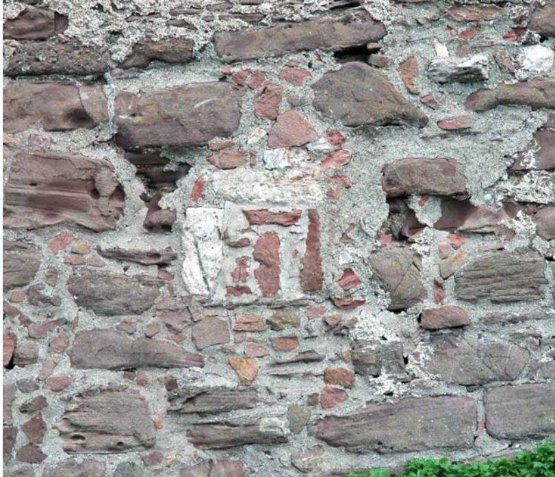
Plate 18: Blocked window into Cellar, WG-2.
