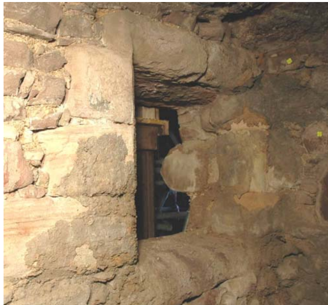
Plate 50: Hatch between passage (F1-4) and Kitchen (R1-5), see the springer stone on the kitchen side of the hatch.
