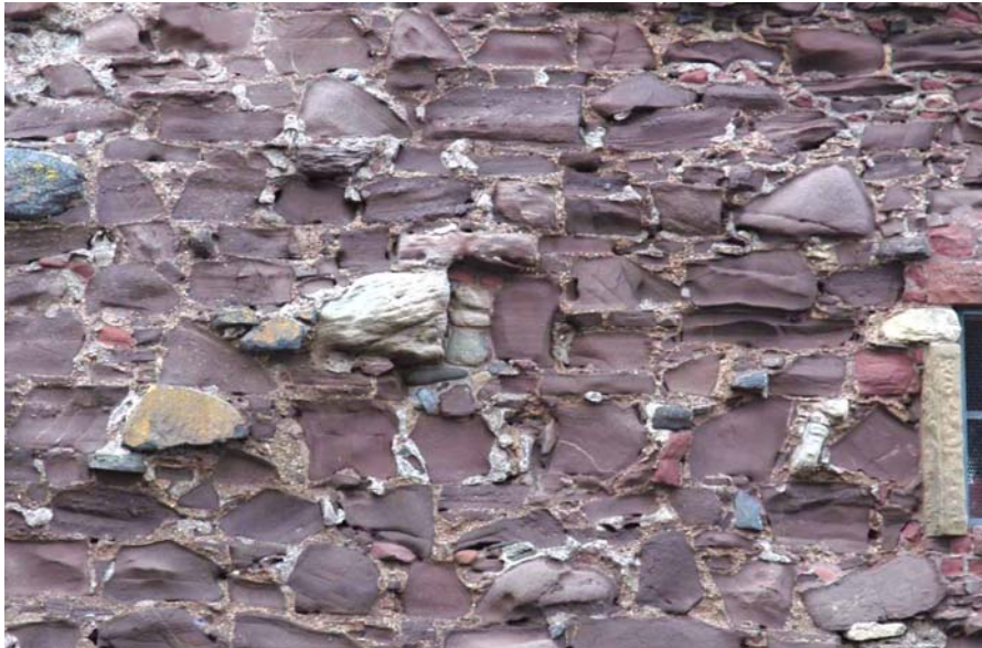
Plate 11: Blocked window WG-4.
